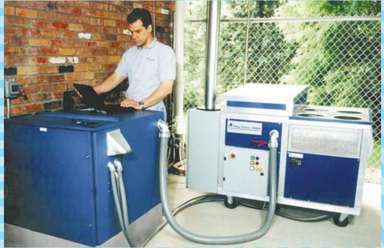
The world's first prototype polymer electrolyte membrane fuel cell (on the right) used to provide all residential power needs for a home in Latham, New York. This 7kW unit is attached to a power conditioner/storage unit that stores excess electricity. (Courtesy: Plug Power)
